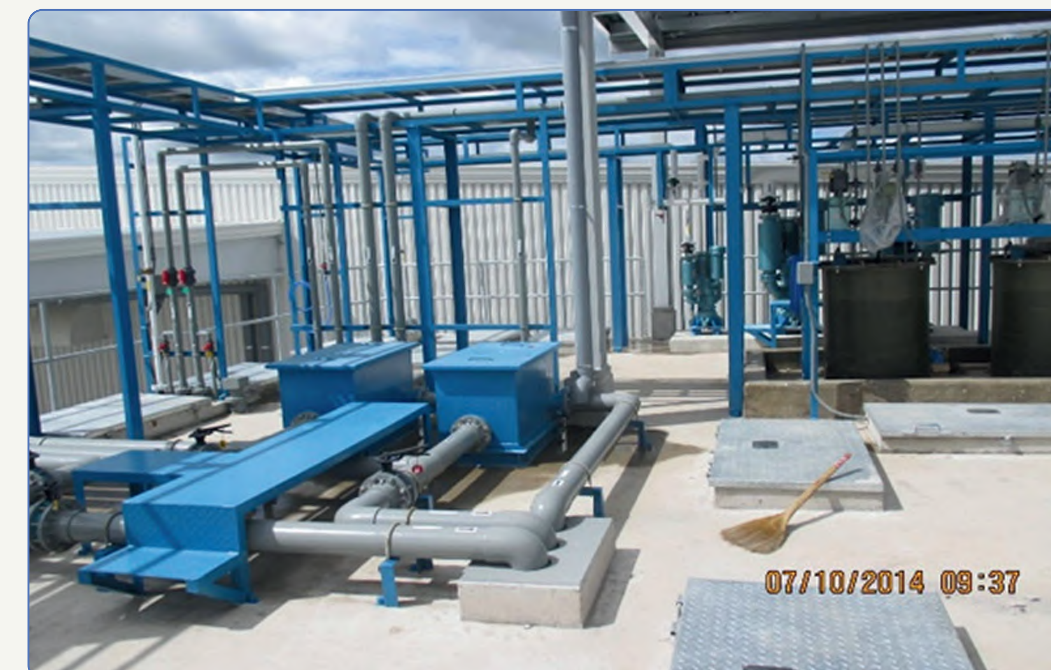
Wastewater Treatment Plant
