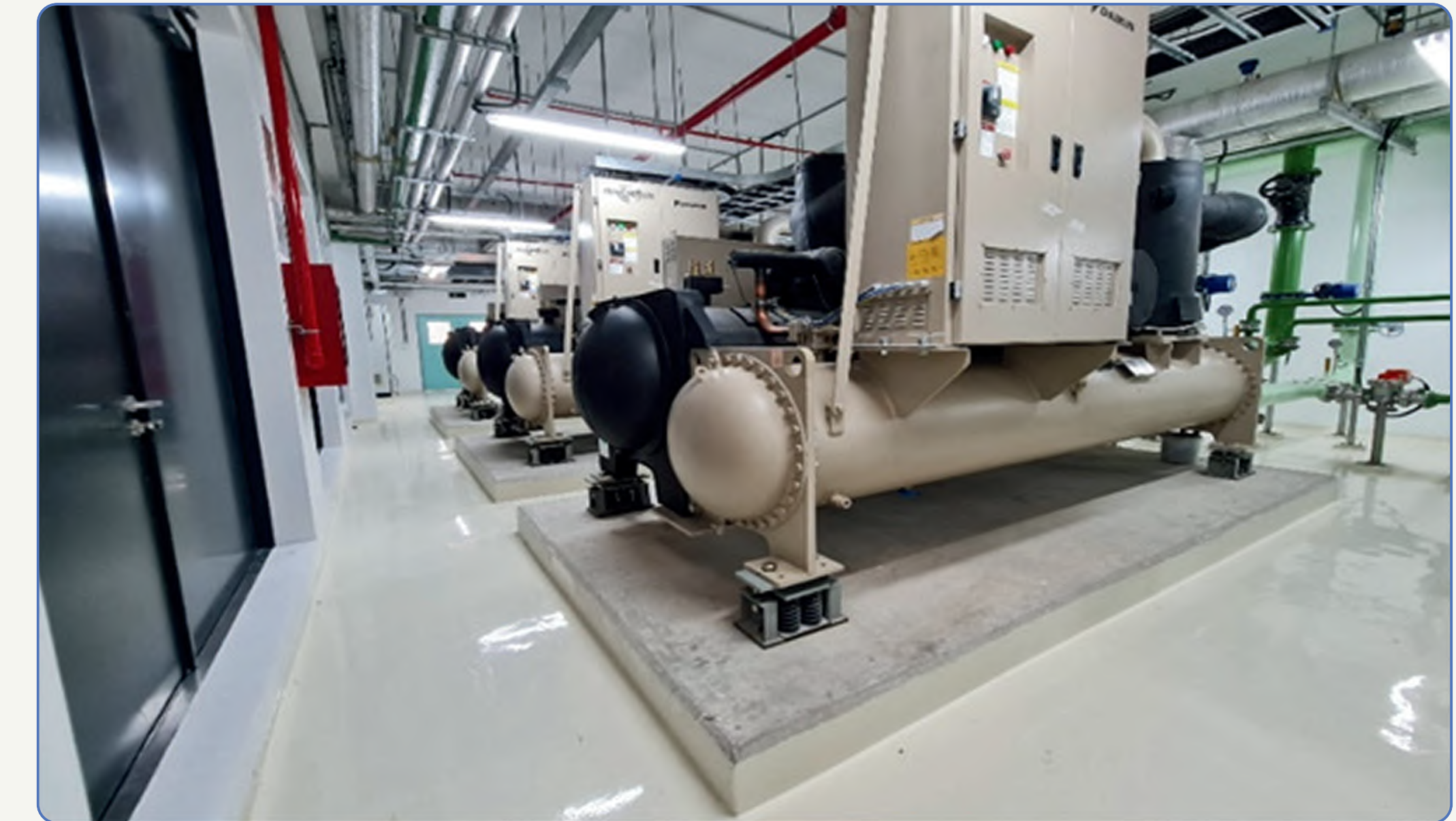
Chiller Plant Room
