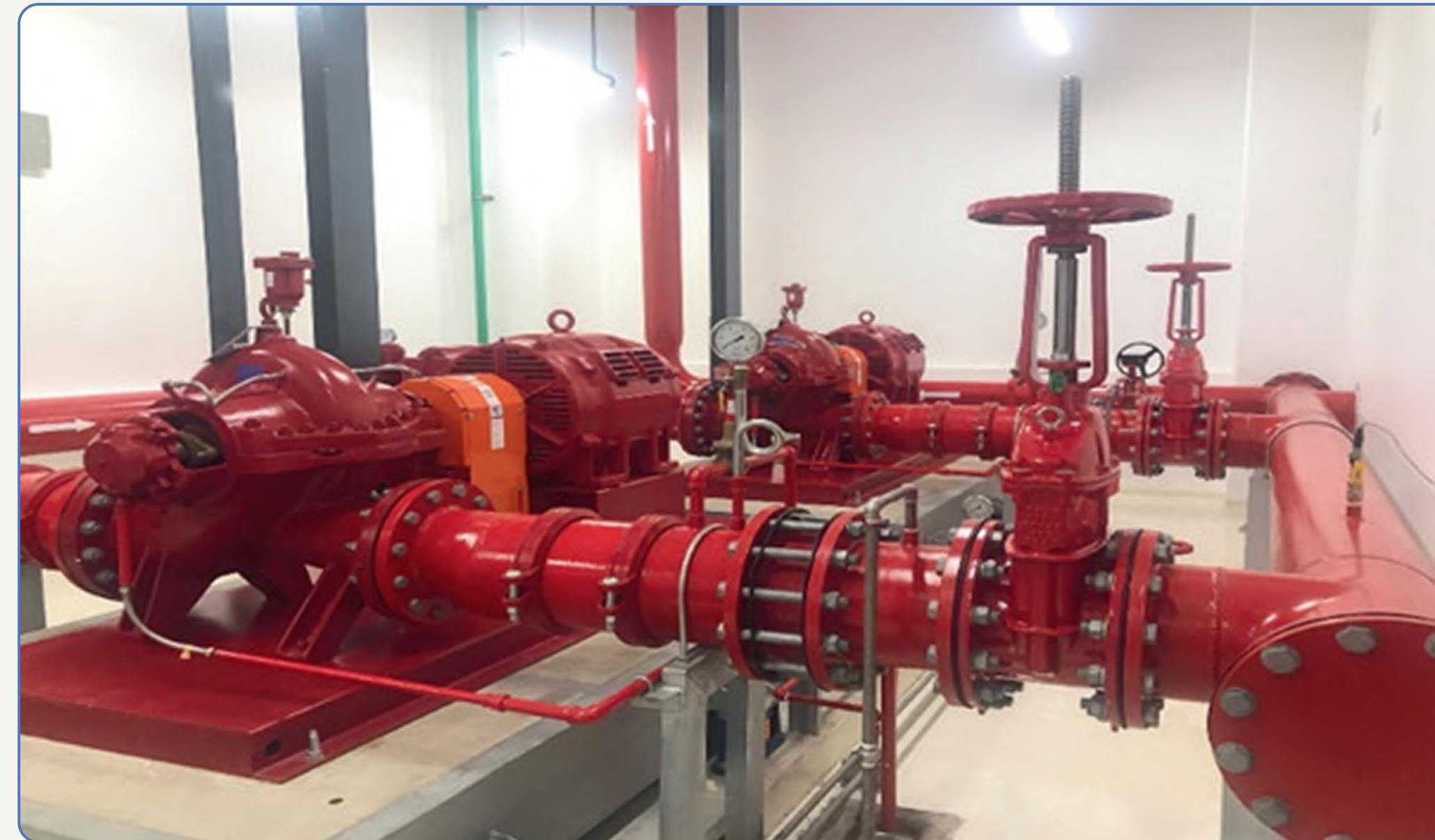
Pump Room Complying with NFPA
