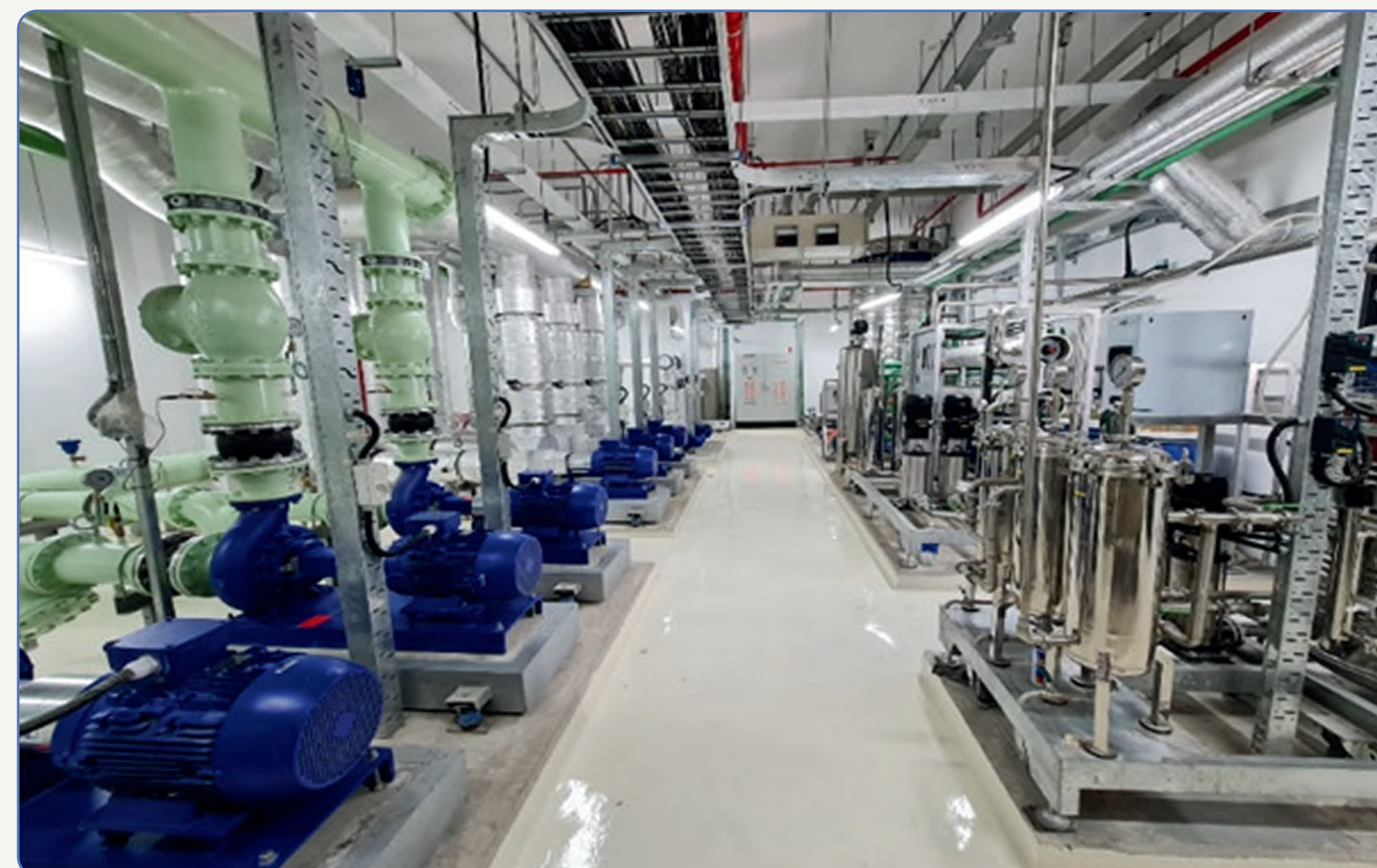
Pump System for Chiller Plant
